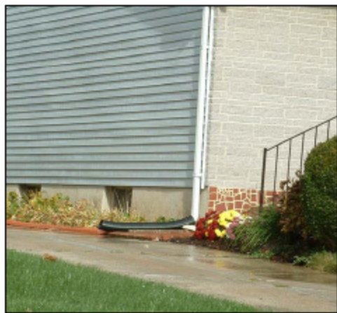
Figure 1: Downspout Intentionally Bypassing Landscaped Area and Draining onto Driveway
