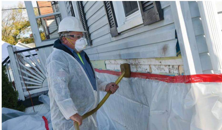
MORPC offers home energy efficiency and safety services at no cost to income-eligible residents to help keep them warmer in the winter and cooler in the summer. The work might include adding home insulation, as seen above.
