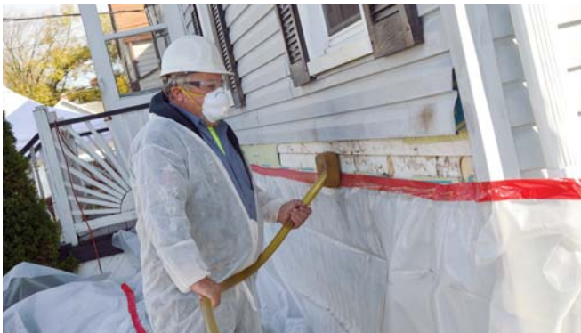
The process of insulating a home is demonstrated at MORPC's annual Home Weatherization Showcase.
