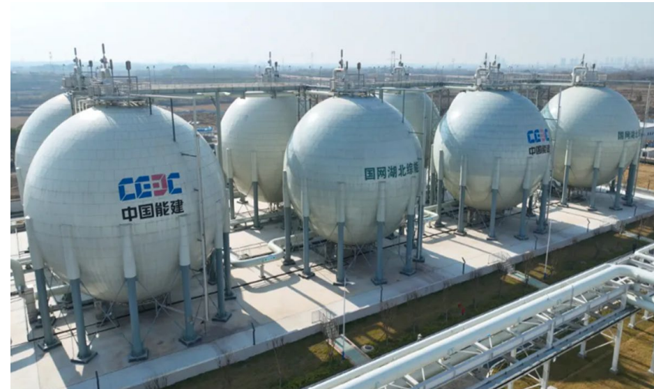
World's first 300 MW CAES in Hubei, China 1.5 GWh, storage volume=24.7M ft 3
