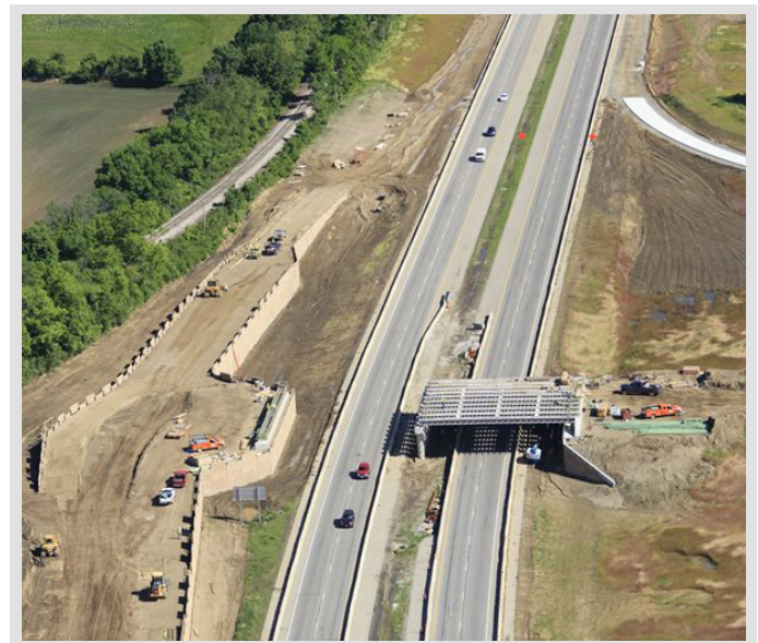
Construction of the recently completed Carroll Interchange at the south end of the corridor
