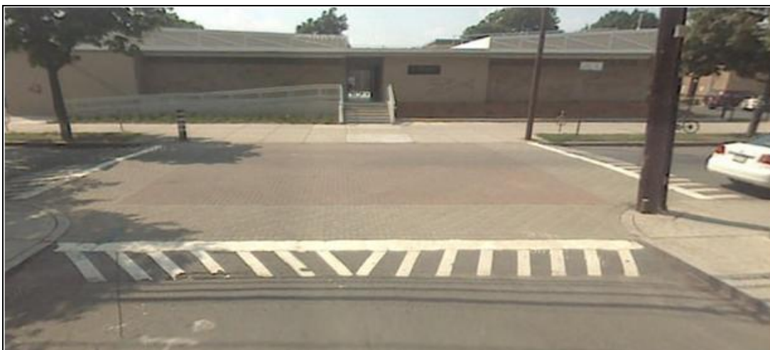
▲ A speed table with warning white stripes and red brick. (Source: Google Maps) • At the intersection of Marcella Street and Berkshire Street in Cambridge, MA.
